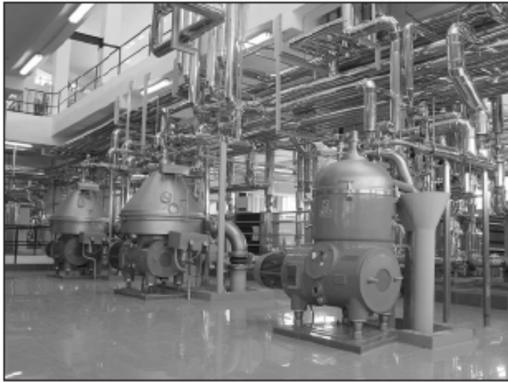
A piping network in an industrial facility.
